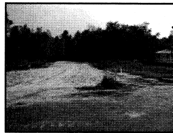
A 21-lot subdivision proposal is pending for this Fairgrounds Road site (left). A home on West Meadow Road is near completion (below left) while work begins on a foundation for a home in a Cressy Road subdivision (below right.)
